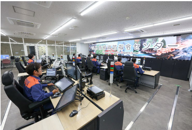
The dispatch room at the Yamaguchi Western Fire Dispatch Center
