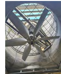
Lightweight plastic fans in cooling tower
