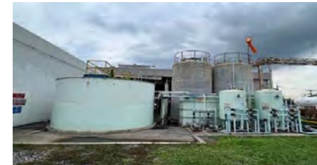
Chemical wastewater processing facilities (FGT)
