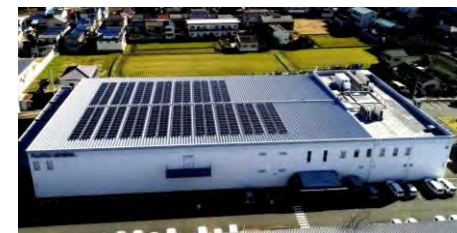
Solar panels on the roof of our Matsubara Office (operation from January 2024)
