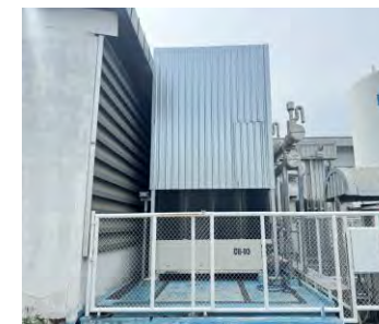
Chiller with stacks
