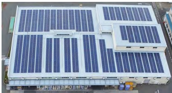
Solar panels (Operation from December 2017)
